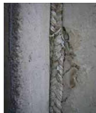
Joints de dilatation
